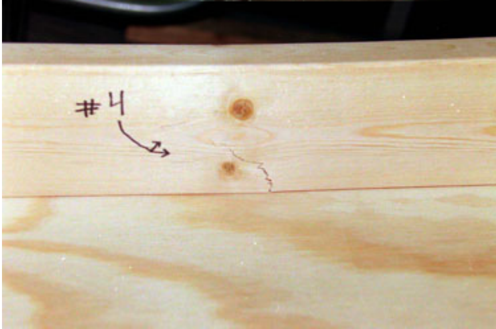
PHOTOGRAPH 27 SPECIMEN 4 FAILURE OF 2 x 4 STUD
