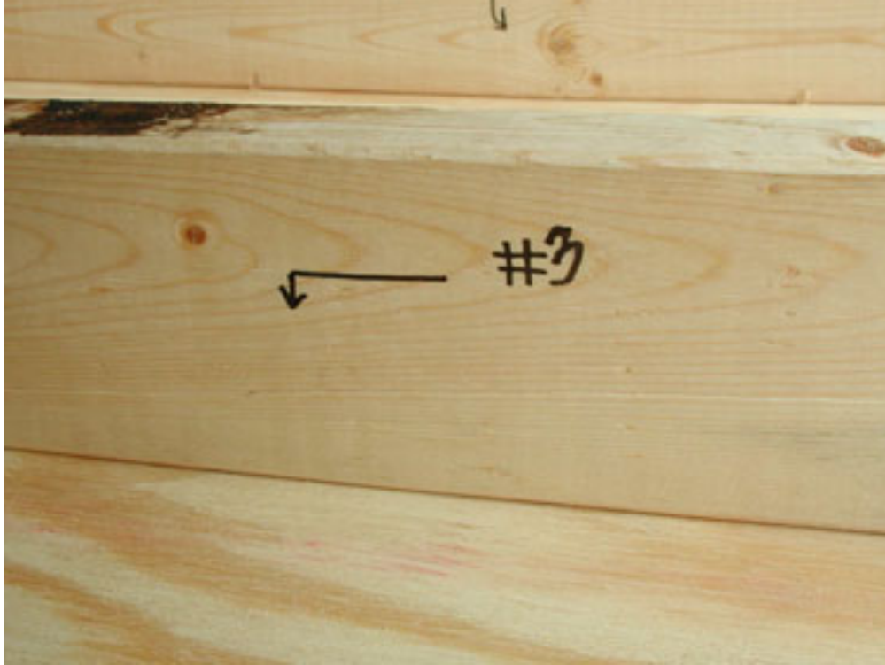
PHOTOGRAPH 23 SPECIMEN 3 FAILURE OF 2 x 4 STUD
