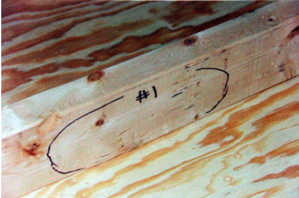
PHOTOGRAPH 19 SPECIMEN 1 FAILURE OF 2 x 4 STUD
